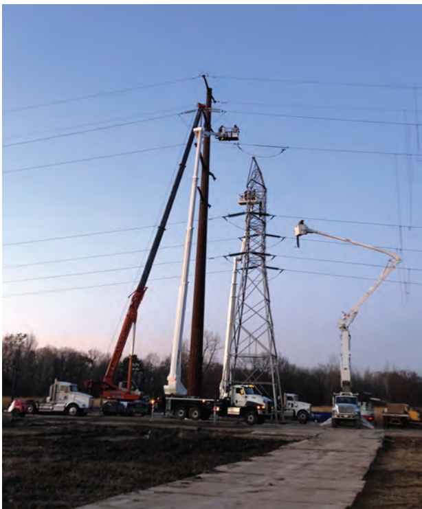
▲ Chris Kirby (2006) is a Senior project Manager with ComEd in Chicago, IL. One of his projects is rebuilding a 138kV Transmission Line through Matthiessen State Park. This project was part of a NERC Compliance Program.
