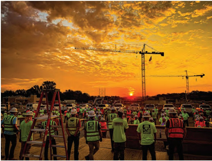
▲ Kerry Klausner (2011) is a Project Manager with McCarthy Building Companies. The picture is a Monday morning (sunrise) safety talk at his Tomahawk Creek Wastewater Treatment Facility project in Kansas City, KS.
