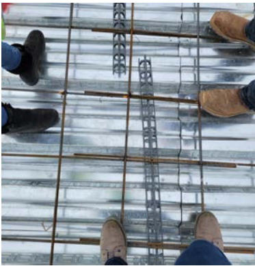
Checking out the chairs and reinforcement for the slab on deck pour
