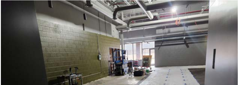
From the high bay looking east at a new informal learning area
